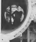
Viewed through the length of an exchanger shell, this workman is using a chipping hammer to clean the inside. He is working at the battlefield (7).
